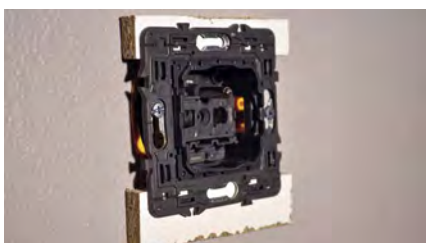
Find the switch.
